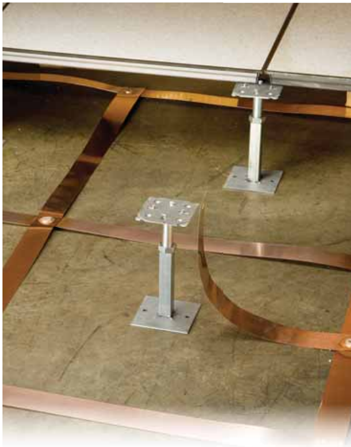
Pre-fabricated Signal Reference Grid installed under computer room floor.
